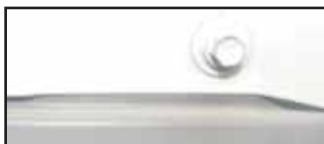
Minimal corrosion is detected along cut end of panel with Edge-Rust Inhibitor application.
