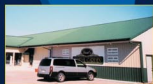
Exposure to UV and elements faded the color of this Si-Poly roof. Add-on roof area at right is original panel color.
