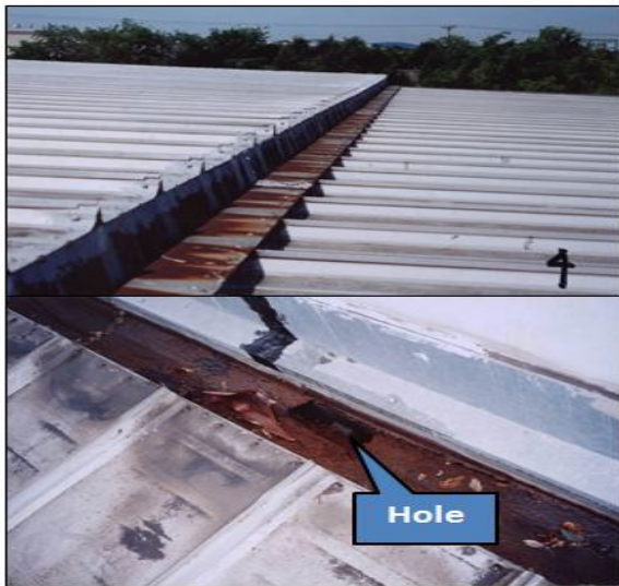
Figure 10-59 Incompatible Gutter, Flashing, and Roof Material
