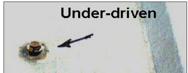
Figure 10-78 Under-Driven Fasteners Will Leak and Corrode
