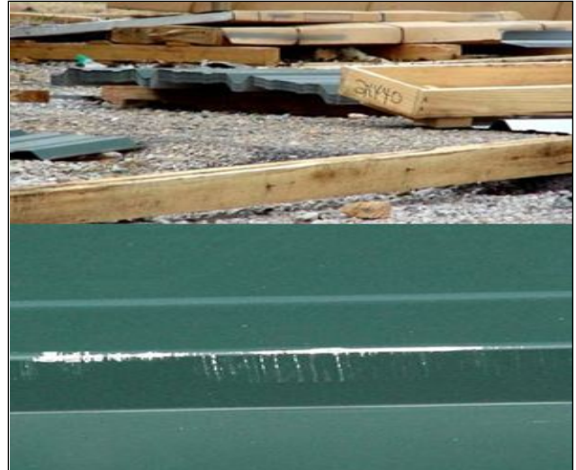
Figure 9-12 Improper Staging of Material Will Cause Damage
