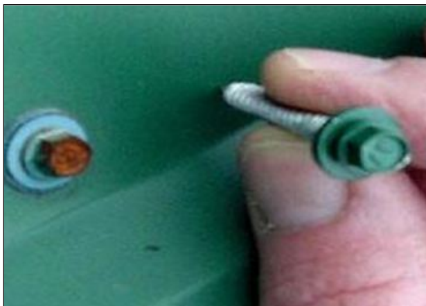
Figure 14-31 Correct Fastener Compared to Installed Fastener
