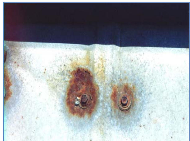
Figure 10-48 Incorrect Fastener Material
