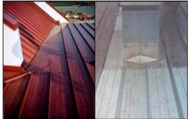
Figure 10-42 Proper Planning and Installation Avoids Ponding Issues
