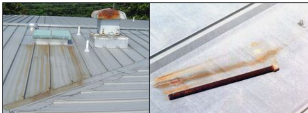
Figure 10-41 Corrosion Damage to a Metal Roof
