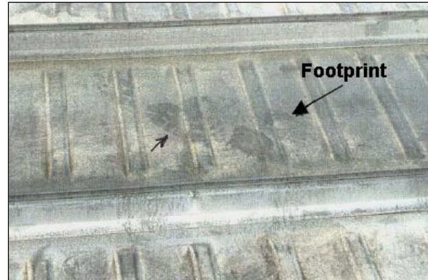
Figure 9-8 Inattention to Footwear May Cause Panel Damage
