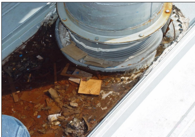
Figure 10-67 Improperly Installed Pipe Blocking Water Flow
