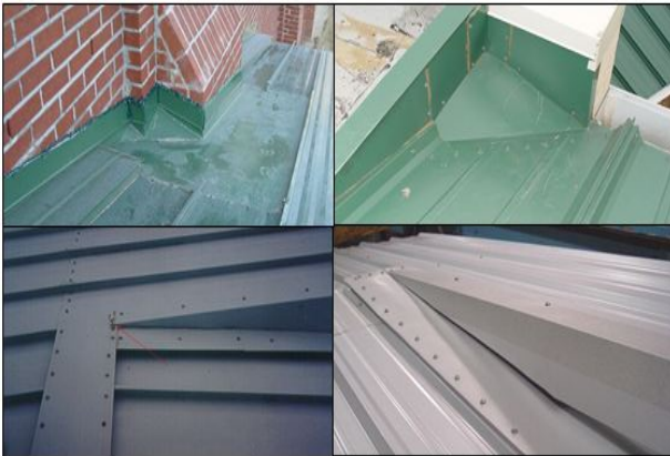
Figure 19-14 Roof to Wall Flashings Vary Widely
