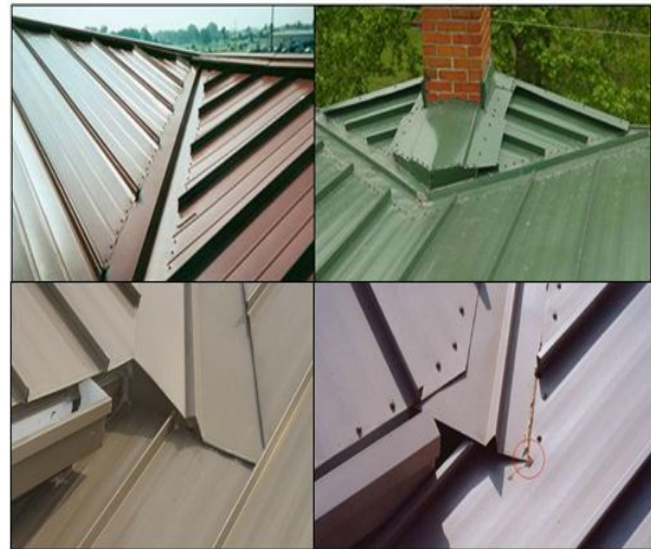
Figure 19-13 Valley Issues Affect Water Flow and Drainage
