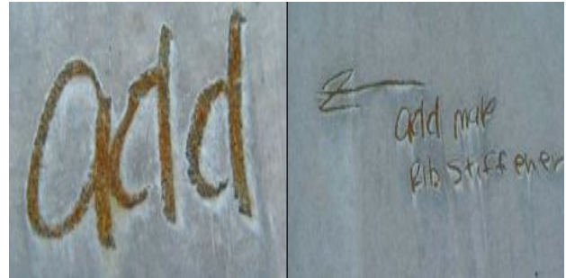
Figure 10-45 Corrosion Caused by Graphite Pencil
