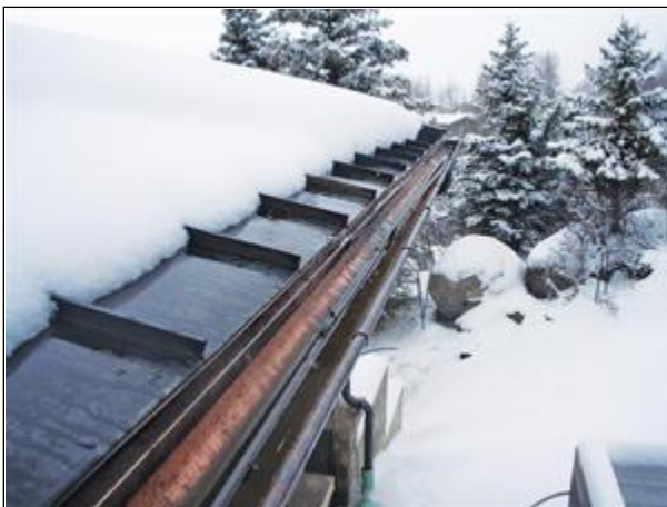
Figure 8-21 Electrical Ice Melt System Installed Along the Fascia Avoids Penetration of the Roof Surface
