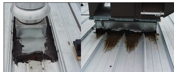
Figure 8-9 Improper Curb Types
