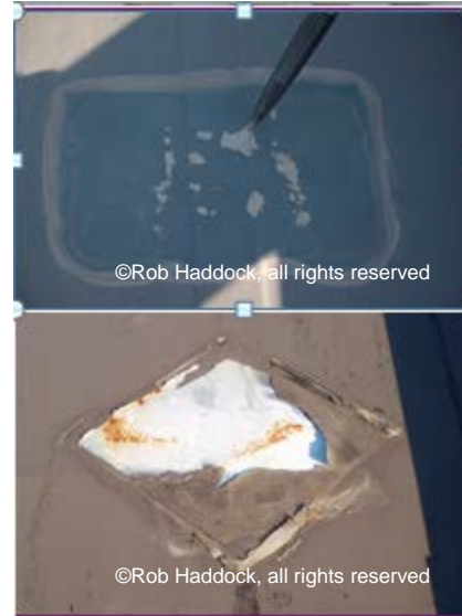
Figure 8-23 Failure of adhesive applied snow retention devices due to inadequate quantity, or design of system, or improper adhesive type, or bonding failure
