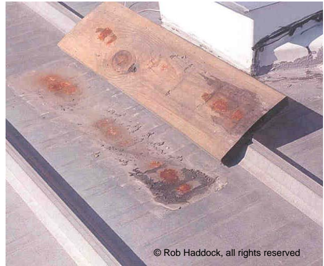
Figure 11-18 Corrosion Caused By Failure to Clean Up After Work Was Performed
