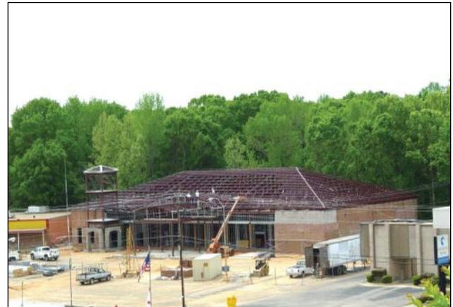
Figure 9-1 The Job Site Itself Presents Many Hazards
