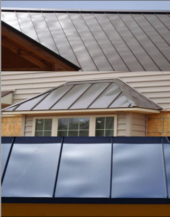
Figure 10-38 Oil Canning of a Metal Roof
