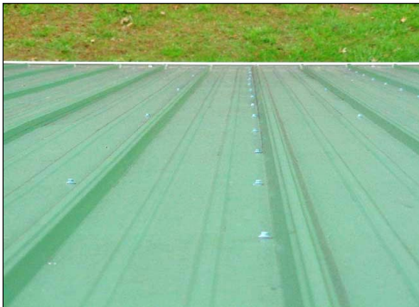
Figure 14-30 Color and Alignment Errors in Fastener Installation are Very Visible
